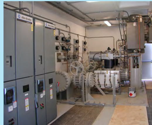
Interior view with pumps set.
